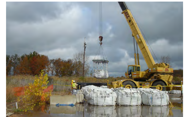
Waste containment bags are loaded onto railcars at the Painesville site near Cleveland.
