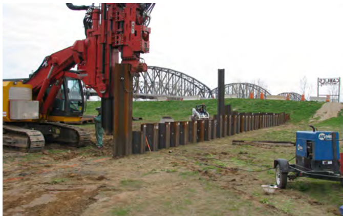
Heavy pile-driving equipment initiates the sheet pile protection for the St. Louis City Vicinity Property at the St. Louis Downtown Site location.
