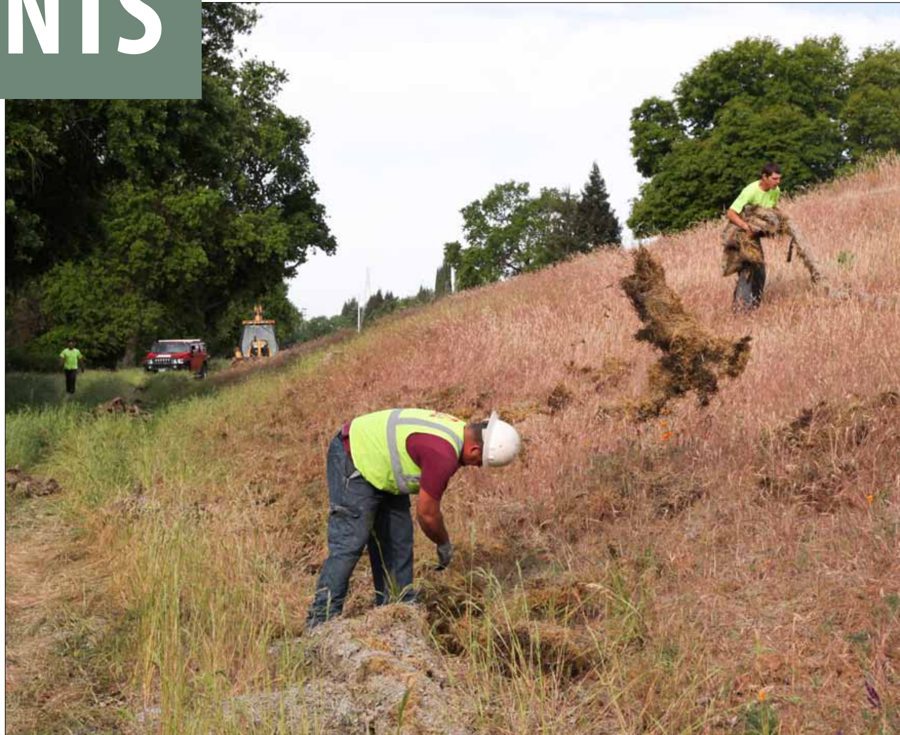
Construction workers for the U.S. Army Corps of Engineers Sacramento District remove decomposed straw-netting April 19 along the American River in Sacramento, Calif. The rolls of straw, called wattles, were put in place to help native grasses take hold on the newly refurbished levee during the winter rains. Their removal is one of the final steps in restoring this reach to its pre-construction condition. More than 4,000 feet of this levee was reinforced and raised an average of 1 foot to safely pass more water coming from Folsom Dam and its auxiliary spillway, currently under construction and slated for completion in October 2017. (U.S. Army photo by Todd Plain)
