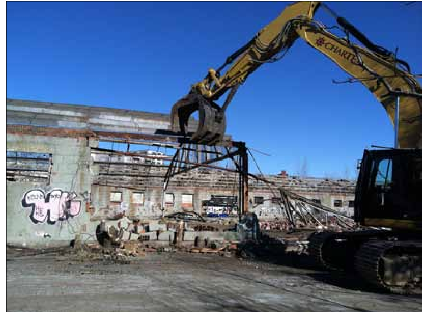
Buildings are demolished as part of the remedial action plan for the Watertown GSA Formerly Used Defense Site. (Photo by Charter Environmental)
