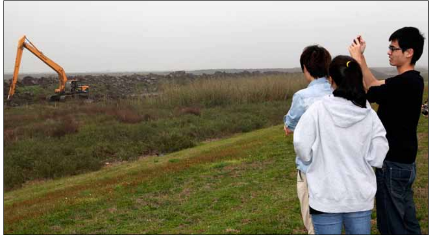
Visiting Louisiana State University students, enrolled in the Robert Reich School of Landscape Architecture, watch a heavy equipment operator work to construct dewatering ditches at the San Jacinto Placement Area to allow for the outflow of excess water and increase the dredging placement area's capacity to hold more dredge material. (Courtesy photo)
