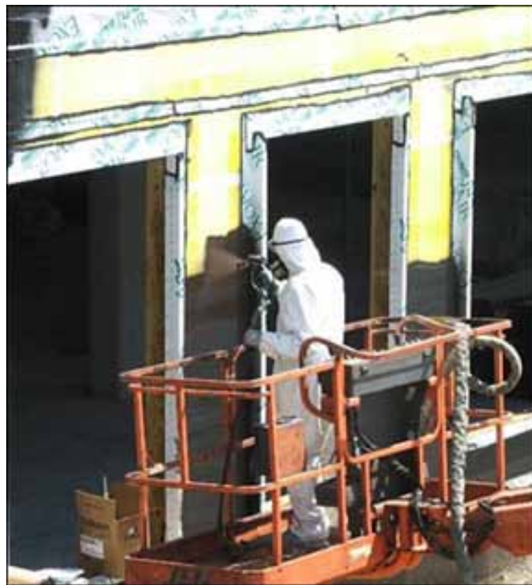
Continuous air barriers like this one being installed can save up to 45 percent on energy costs. (Courtesy photo)
