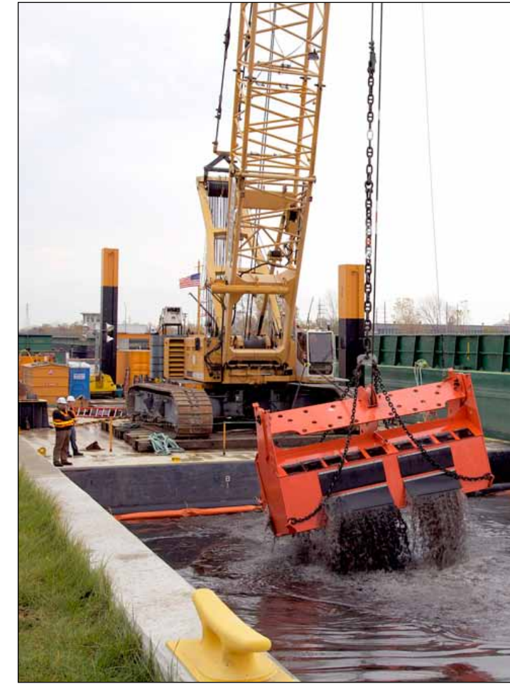
Sediment is removed from Indiana Harbor and Canal, for the first time in 40 years on Oct. 23. (Photo by Jessica Majchrowski)
